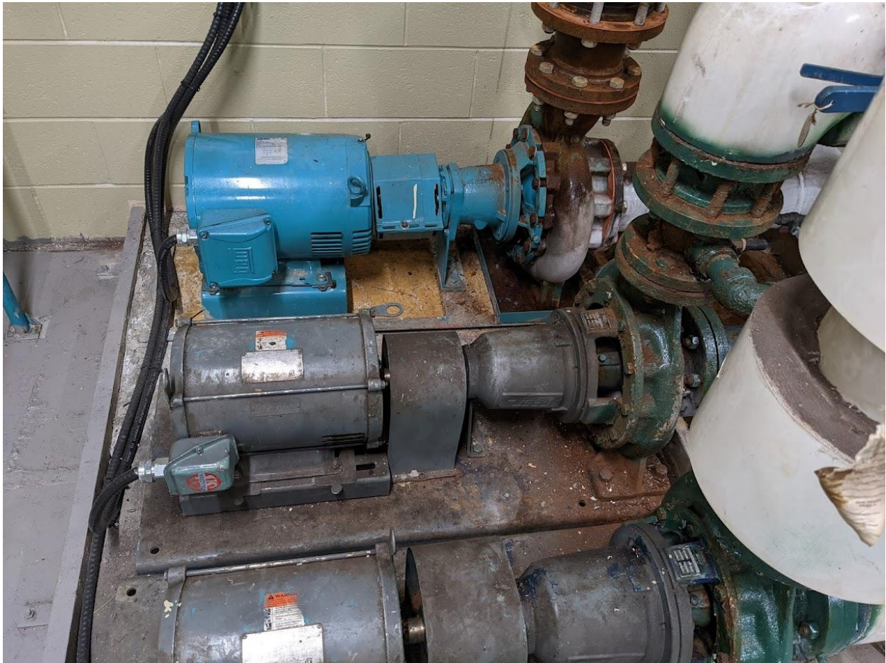
Curling Pump – Center – To be replaced
